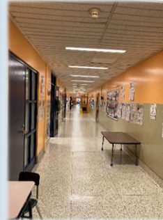
Marzolf Primary School -Sagging Lay-in Ceilings.
