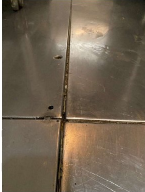
Walk-in cooler/freezer floors. The floor panel delamination and joint degradation occurring on both the ceiling and wall panels.
