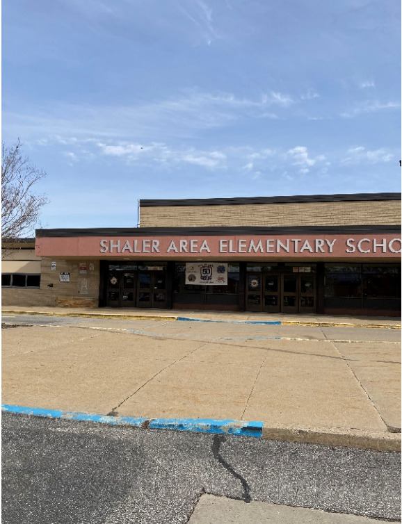
Concrete walkways are in poor condition. Building entrance and walkways are not protected from vehicles driving off the asphalt.
