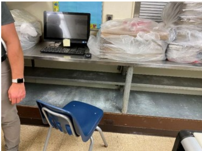
Kitchen serving /cashier window undersized.
