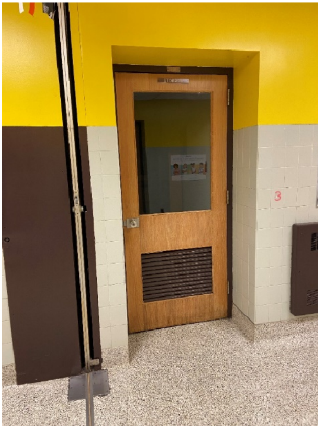
Typical Non-compliant Interior door -do not provide accessible clearances.
