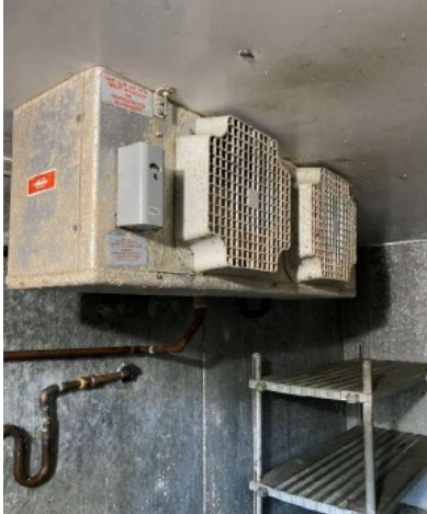
Interior of Walk-in Cooler.
