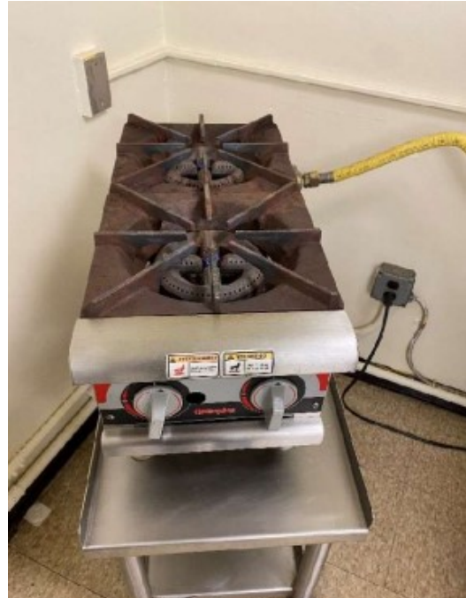
Gas Appliance Not Vented or Protected by Fire Suppression or Fire/Fuel Shut-off.
