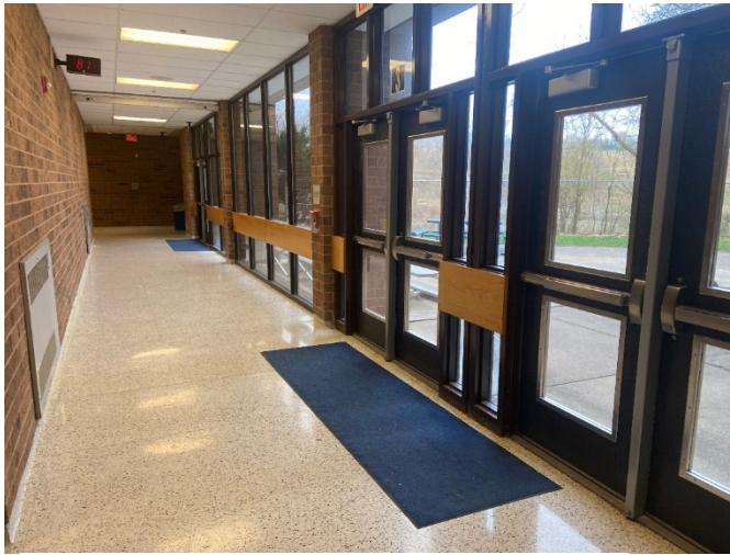
Main aluminum entrance doors need to be replaced.
