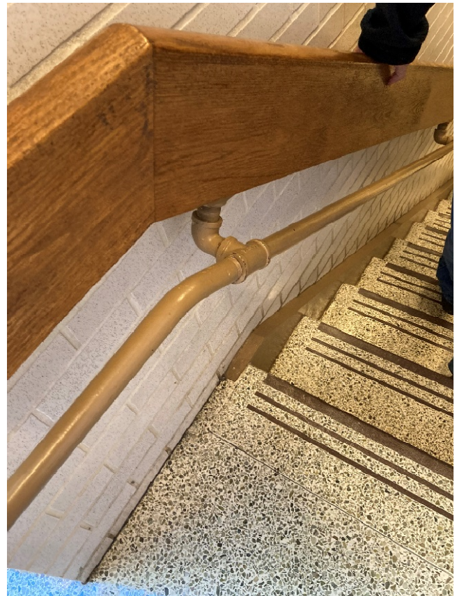
Stair's handrail is non-compliant per ADA requirements.
