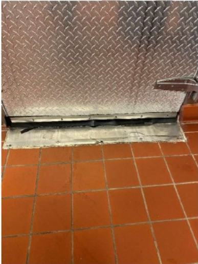
Water Pooling at Exterior of Walk-in Doors.
