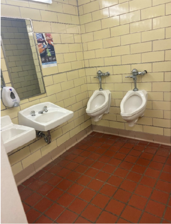
Renovate all building restrooms to provide adequate clearances for handicap; replace plumbing fixtures and accessories.
