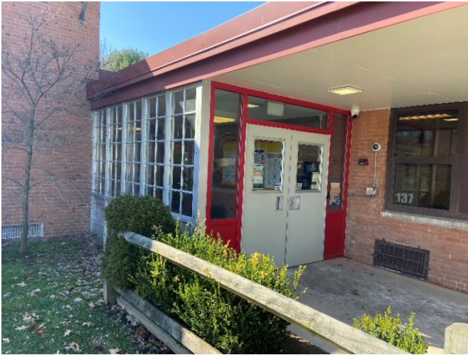
Burchfield Primary – Main entrance storefront leak air and water.
