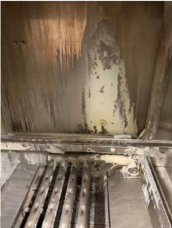
Interior of Dish machine.
