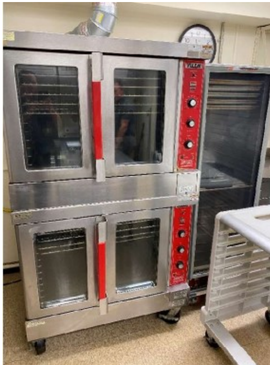
Gas Oven Direct Vented without Fire/Fuel Shut-off or Fire Suppression.
