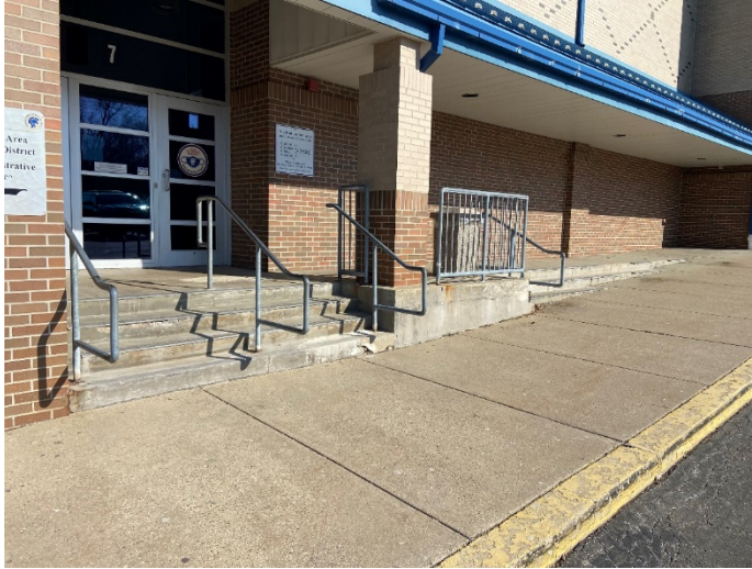
Shaler Middle school –Entrance stairs with metal inserts are in poor condition.
