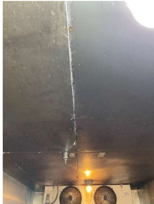
Walk-in cooler /freezer Ceilings.
