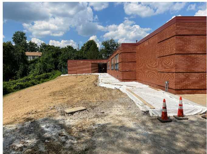
Existing play area being removed to receive new grass and sidewalks to
