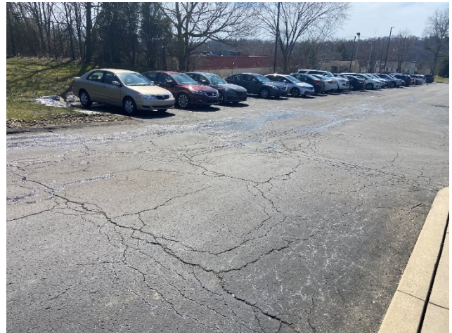
Existing parking lot showing signs of cracking in the front and rear lots.
