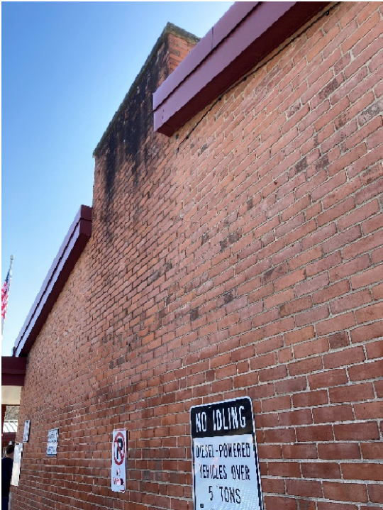
Brick Veneer / Mortar joints damaged due to water infiltration.
