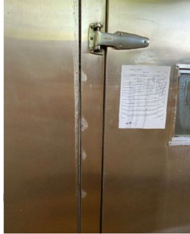
Condensation at degraded Walk-in Seam.
