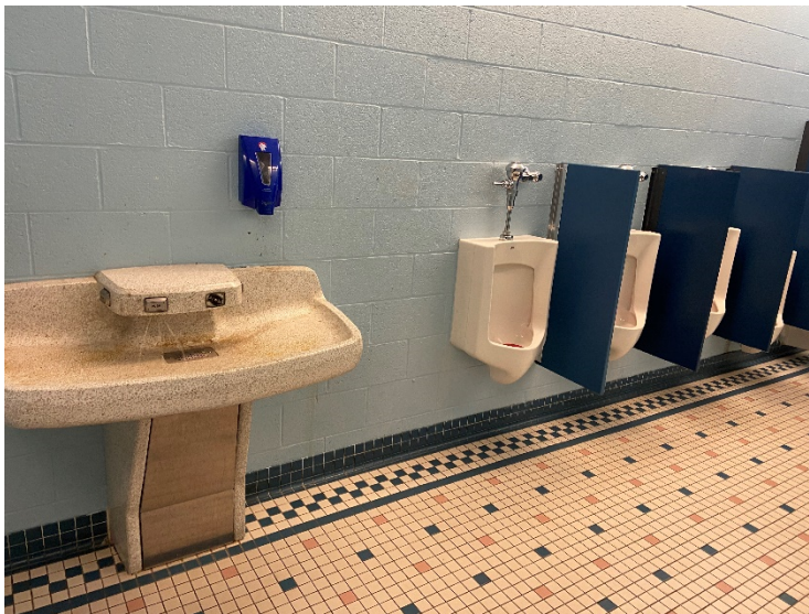
Gang toilet room plumbing fixtures appear to not meet ADA requirements, some have damaged, and corroded manual valves.
