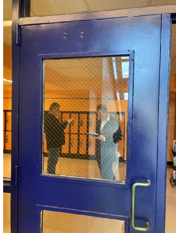
New hardware with lever type are required to meet ADA requirements.
