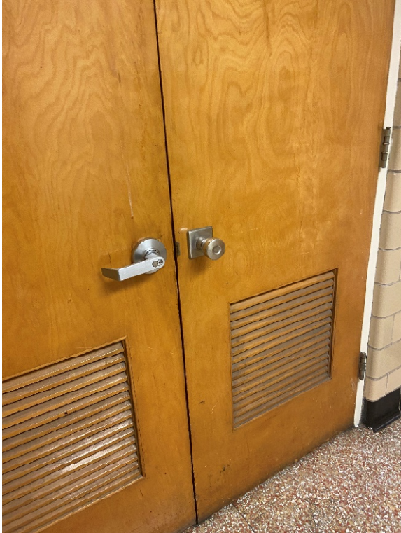
Replace non-compliant door hardware on interior doors with new lever-type locksets and panic devices at exit egress doors.
