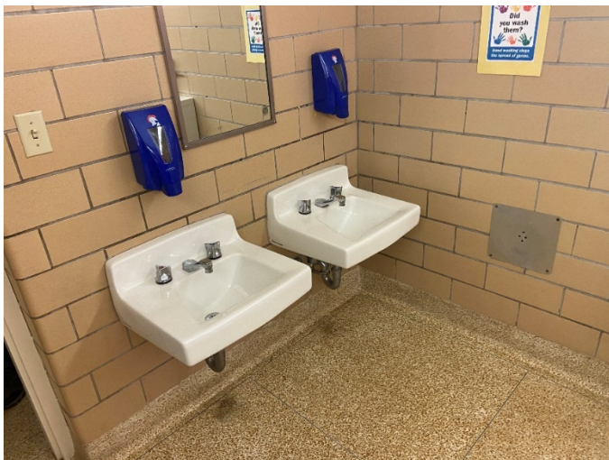
Existing lavatory fixtures do not meet ADA requirements.
