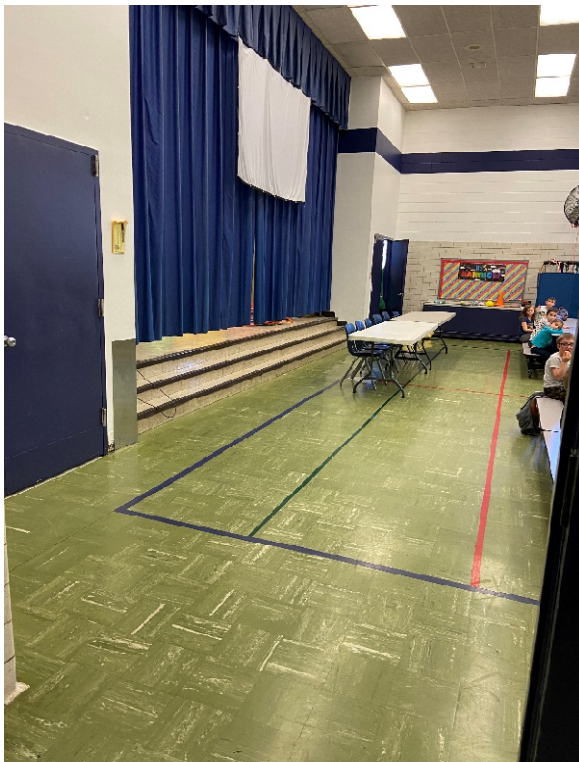
Gymnasium/ Cafeteria- Existing stage level is not ADA compliant.
