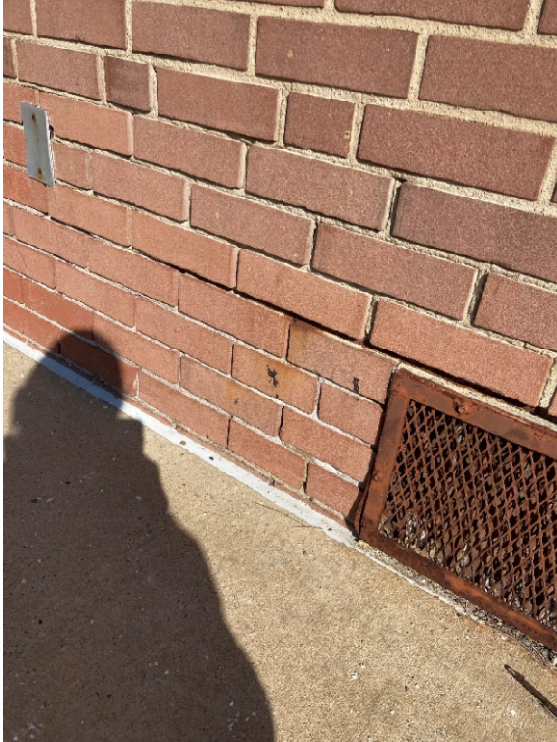
Exterior walls deteriorating due to exposure to weather.
