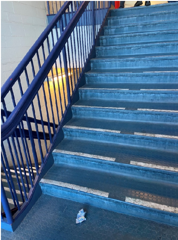
Existing Tread and risers are original and need replacement.
