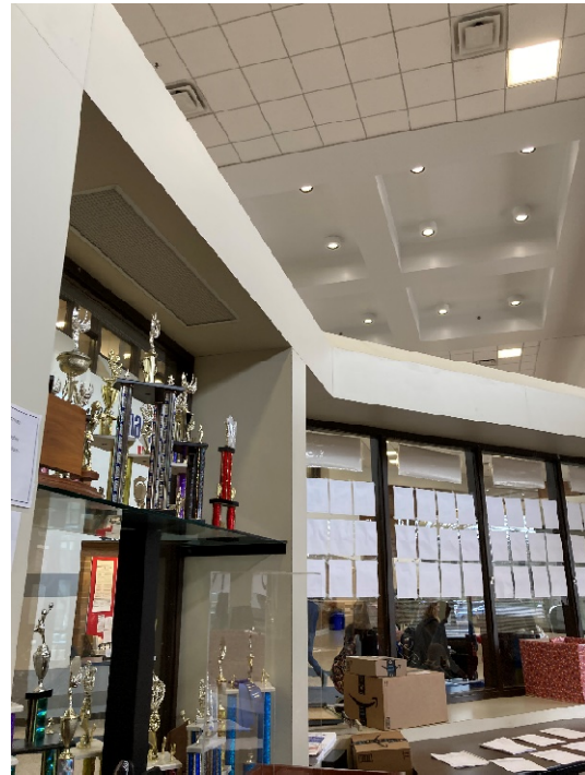
Lobby administration /guidance areas have acoustical issues through ceiling that need to be addressed.
