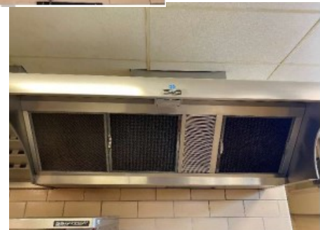
Type 2 Hoods without Fire Suppression Being Used Above Gas Fired Cooking Appliances.
