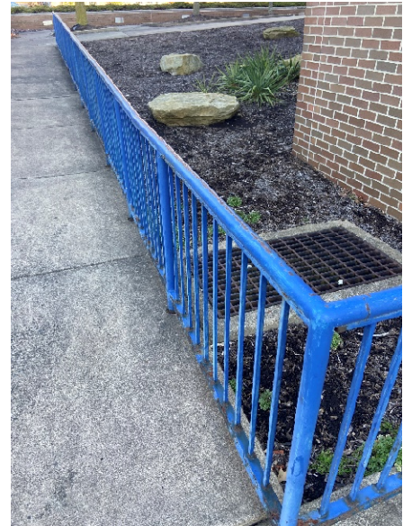
Existing site railings have paint chipping, rusting and require painting
