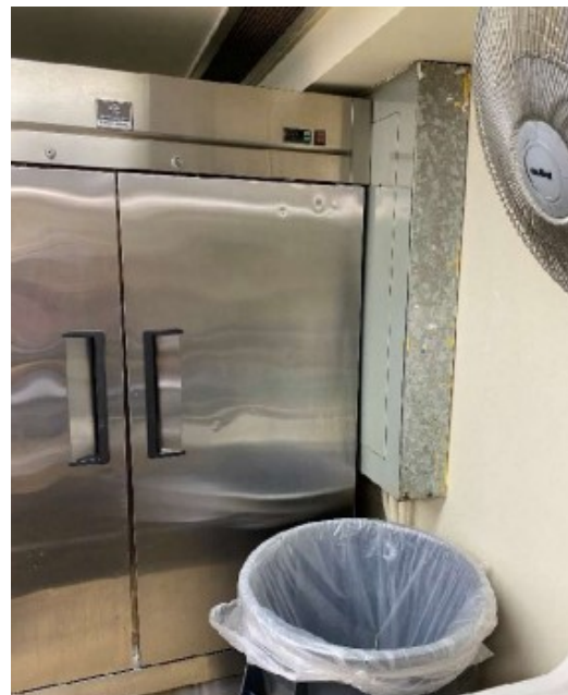
Refrigeration Unit Blocking Elec. Panel.
