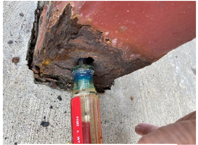
Canopy Column base Deteriorating at Sidewalk.
