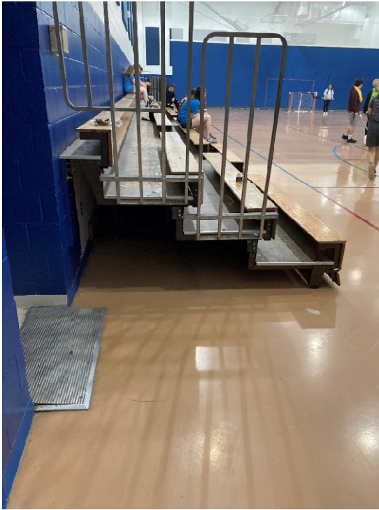
Existing bleachers are in poor condition.
