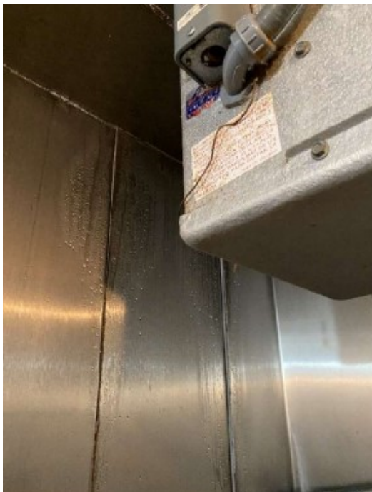
Condensation occurring Inside Walk-ins.
