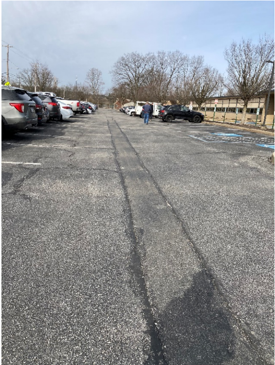
Asphalt in driveways is showing signs of cracking in the front.
