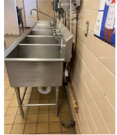
Exposed Plumbing and Gap at Rear of Sink.
